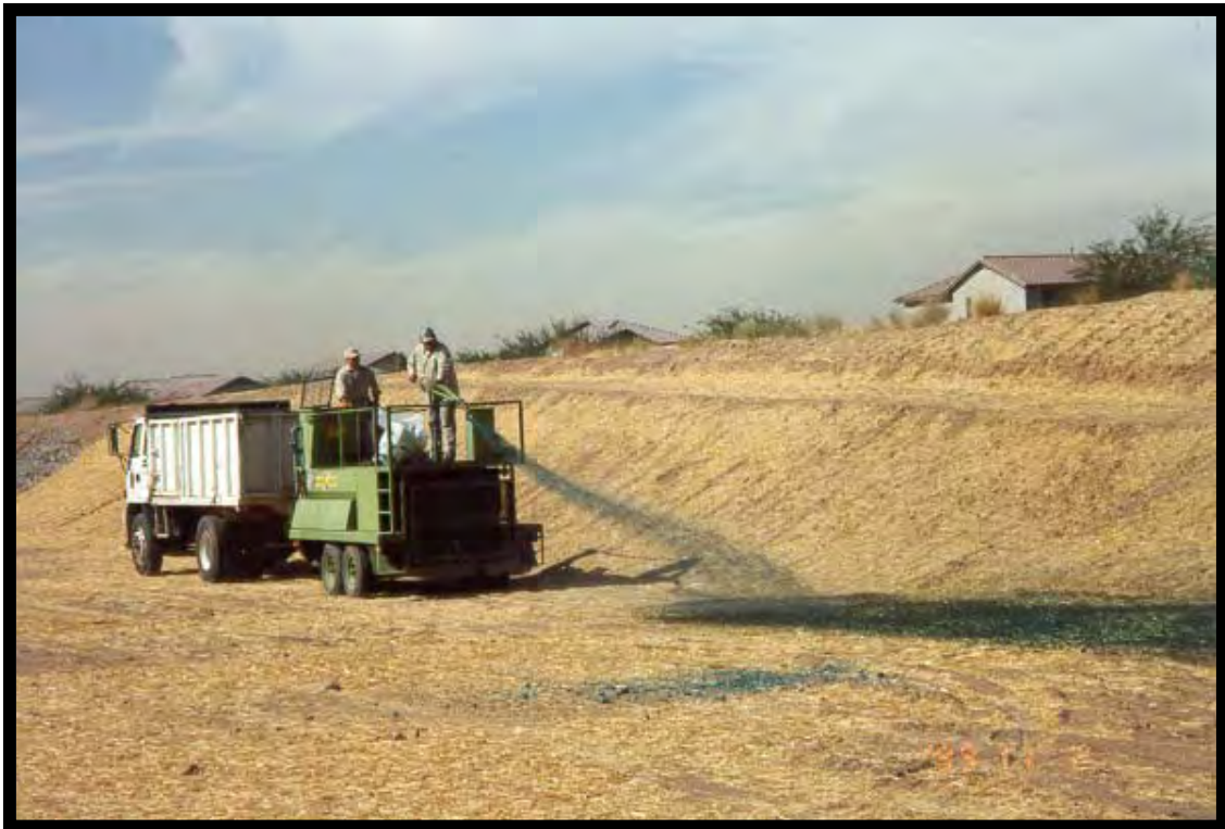
Figure 8. Hydro-seeding operations on a floodway dam in Maricopa County, Arizona (Renckly & Drake, 1999).
