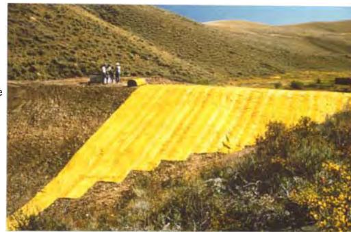
Figure 3. Installed chemical barrier on a dam in Montana (Kershner, 1992)
